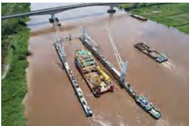
Floating dock in operation
